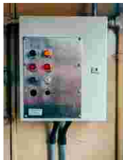
The guard's CDL control panel
