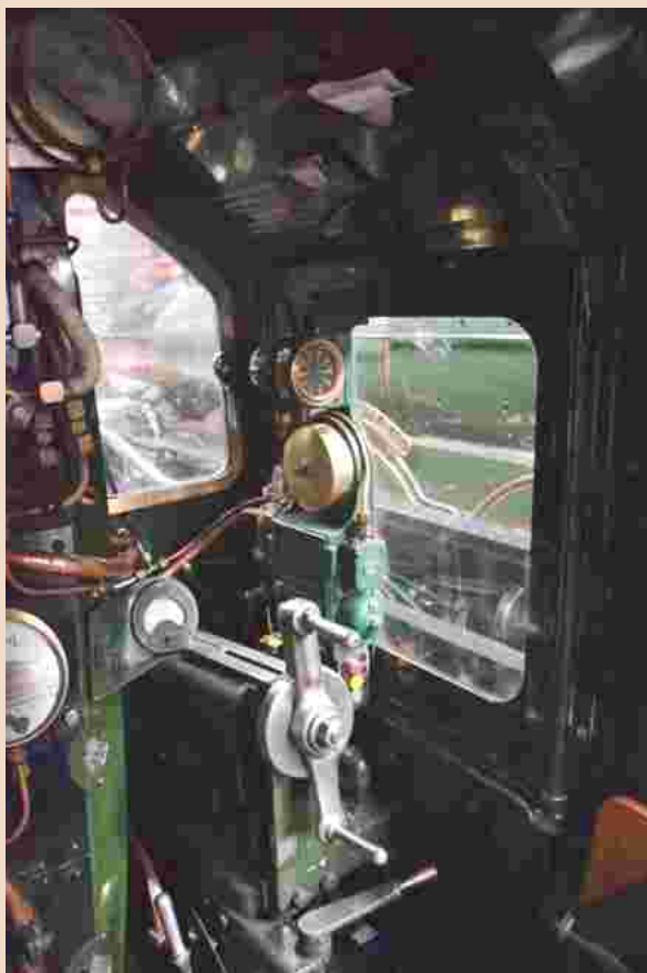
AWS equipment on Clun Castle
